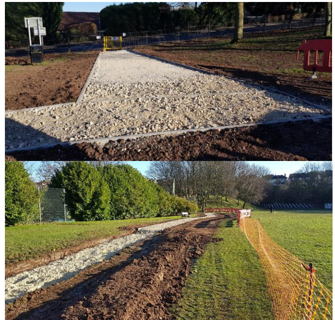
Construction works of the new entrance and footpath from Breck Hill Road January 2024 (works in progress)
